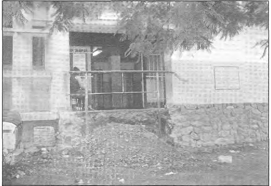
The hospital main entrance affords easy access for the disabled - NOT!
